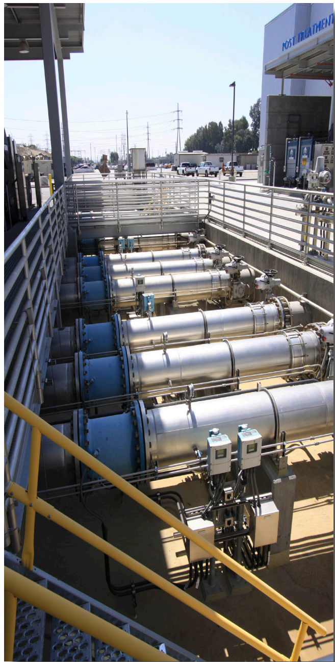
OCWD Groundwater Replenishment System Located in Fountain Valley
